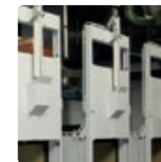
Pneumatic lifting door
